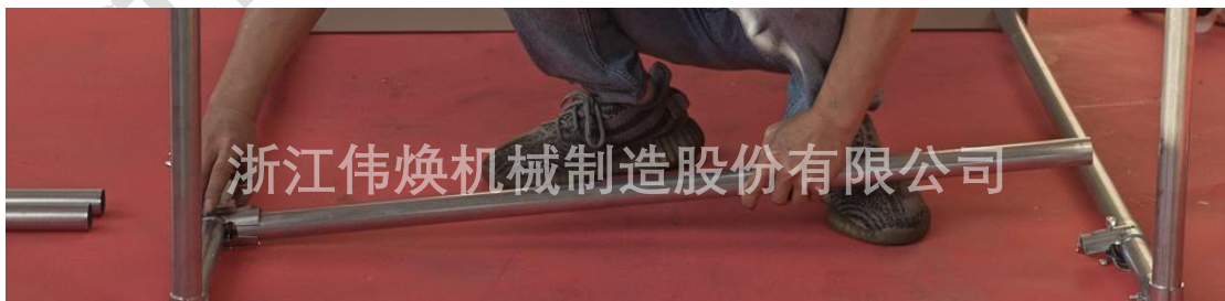
拿出一根钢管连接在直包箍下方，另一根钢管连接在下方钢管 176cm 标记处 connect a pipe under the position of straight hoop, connect another pipe on the position of 176cm marks
